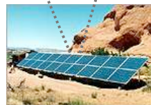
Set of solar panels
