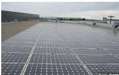
Solar panels on Microsoft building
