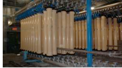
Microfiltration water plant, Petrolia, PA
